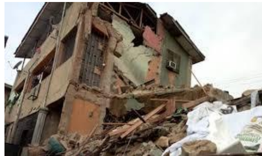
Figure 1. Poor design and specification Source: (Agwuncha 2020)
