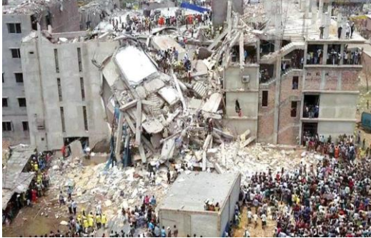
Figure 7. Synagogue building collapse Source: (Olaiya 2016)
