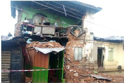
Figure 4. Building collapse in Kaduna Source: (Biniyat 2013)
